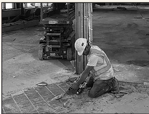
Jerry Garrett of McGough Construction removes grout used to level the Cultural Heritage Center lobby.
