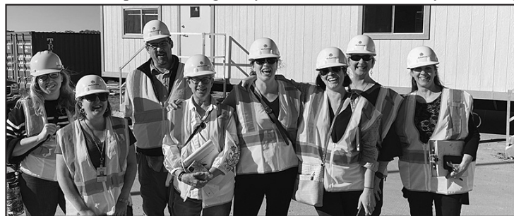
Museum exhibit team composed of staff and contractors visit the construction site of the Cultural Heritage Center under renovation. Pictured (L to R) Corey Christianson, Katy Schmidt, Dan Moeckly, Kate Cravens, Margaret Lee, Amanda Wambach, Catherine Forsch, and Carrie Petersen. Taken 19 Oct. 2023.
